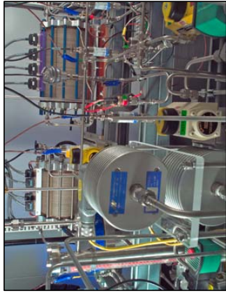
Energy Storage: Developing lithium-ion batteries and regenerative fuel cells to power lunar surface systems.
